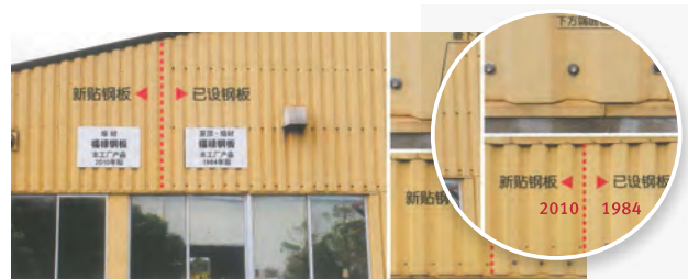
Outer walls of an R&D building for a steel plate factory in Japan (28 years after installation)
